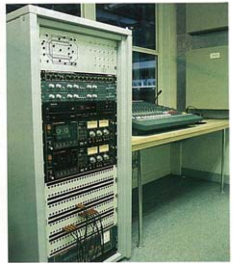
The control end of the system.
